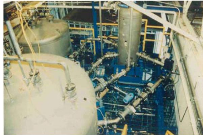
PUMA facility (Top view)
