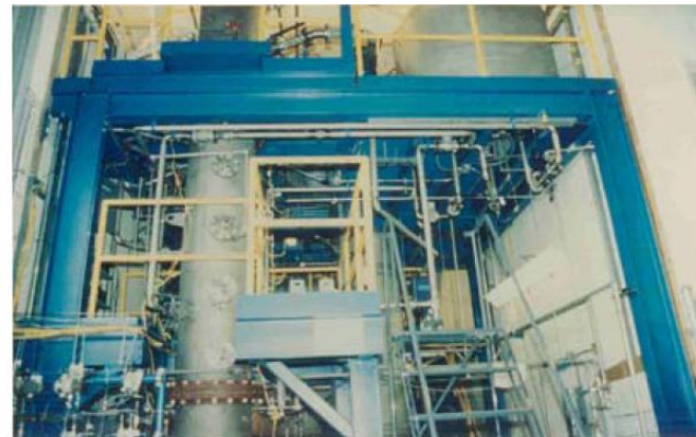
PUMA facility (Front view)
